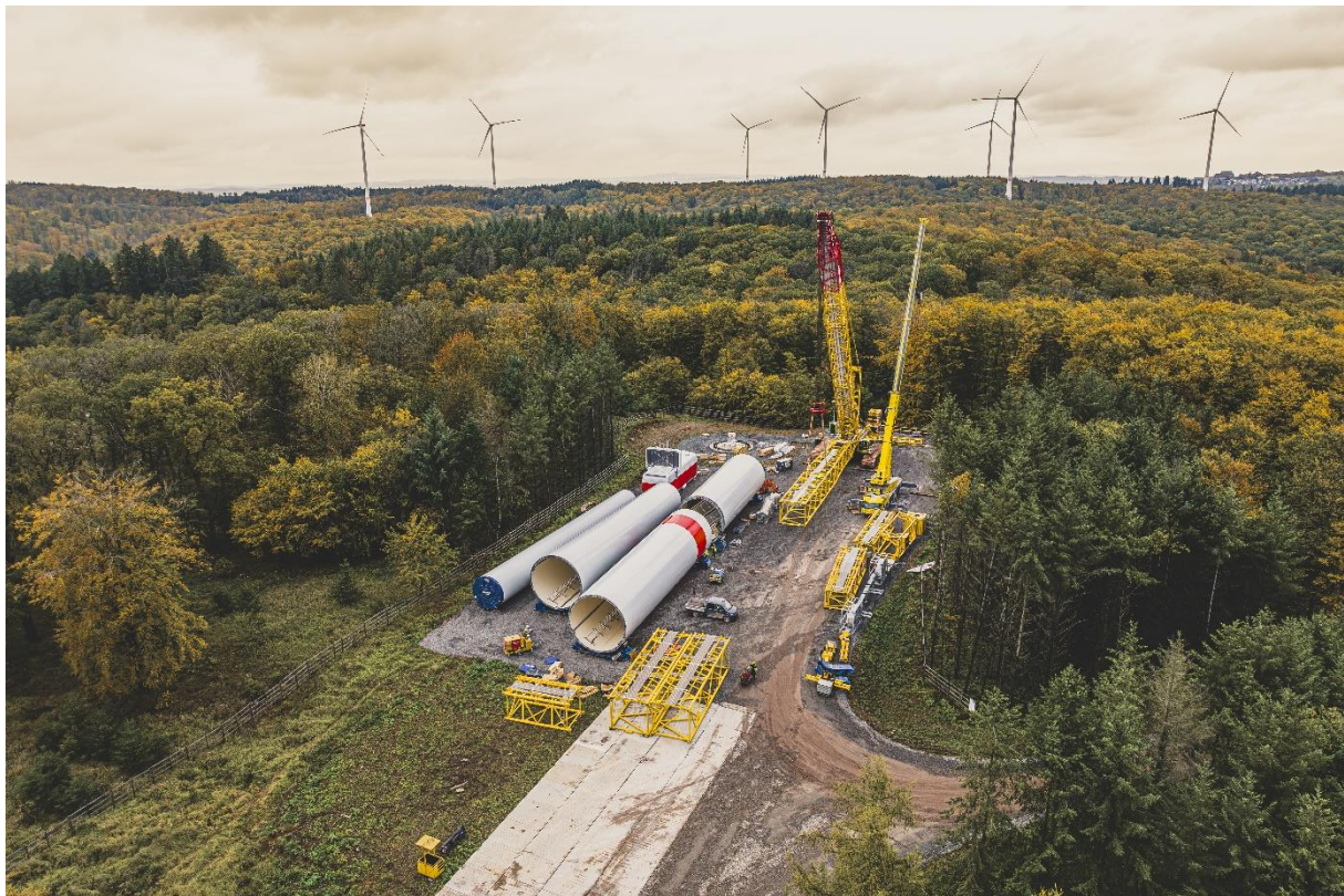
Caption: A specialized crane is used to assemble the wind turbine components, which weigh several tons / Source: Koehler Group
